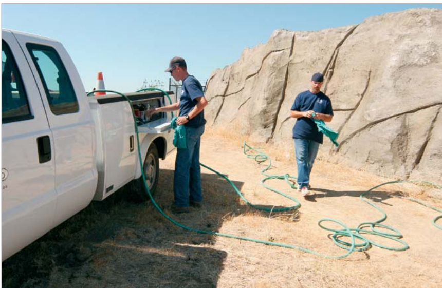
Graffiti Proofer Anti-Stick from SEI Chemical was applied to the rock facade surrounding Brentwood’s new water tank in a one-time spray.
