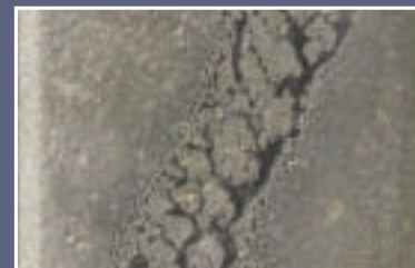
Use on concrete paint cannot adhere and runs off
